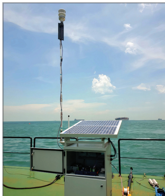
Figure 3: Datalogger, meteorological and current sensors are powered by solar power.
